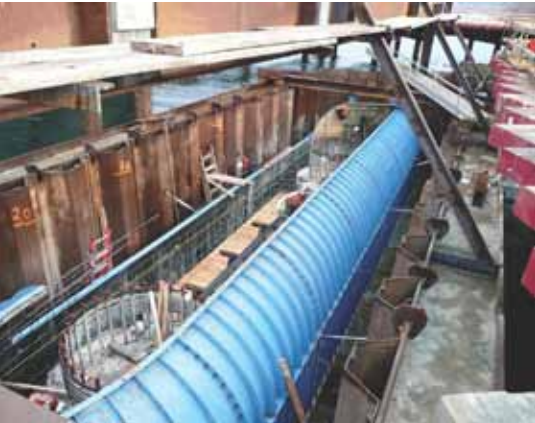
Stage 1 construction utilizing reusable steel footing form. Photo: K. Pope, T.Y. Lin International.
